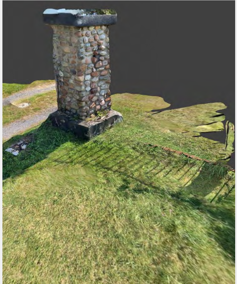
Fig. 9: Missing metal fencing, only shadows captured. Detail of Area mesh scan. Chapel Hill Cemetery, Parishville, NY. HYPERLINK "https://scaniverse.com/scan/nyucimt4ebssjqih" https://scaniverse.com/scan/nyucimt4ebssjqih .
