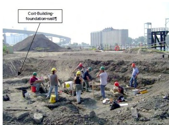
Photograph 2: Erie Canal Harbor site during excavations; Buffalo Creek/Harbor is visible in the background (Panamerican Consultants, Inc., 2005).
